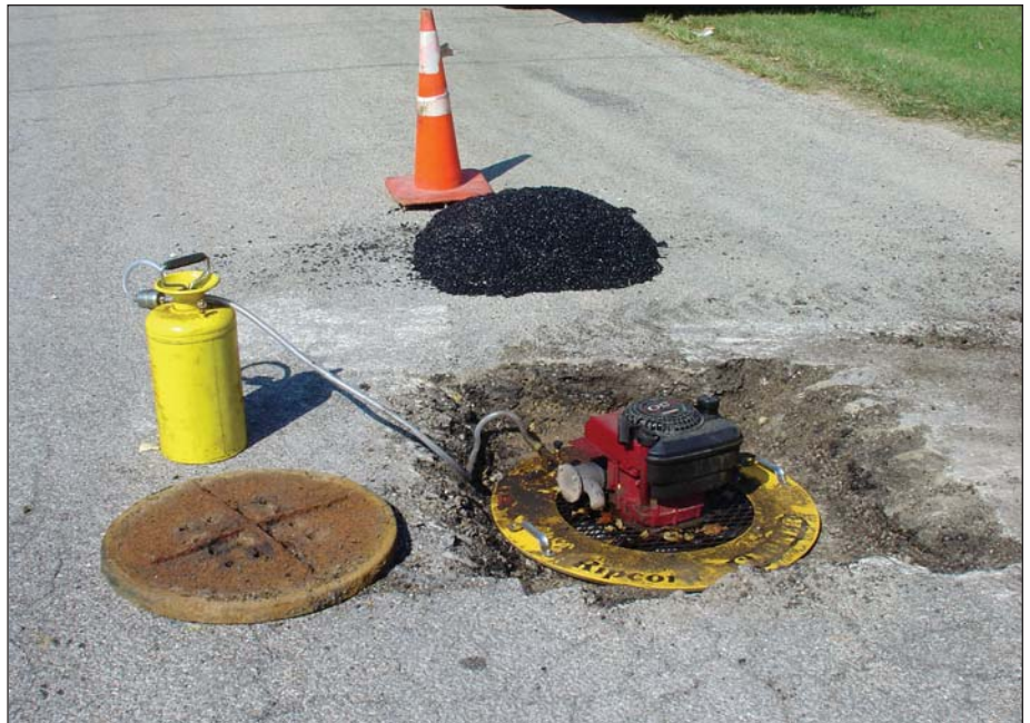
This photo shows one of several "smokers" that KRWA uses to smoke test sanitary sewer systems. The smoker consists of a gasoline engine and high speed fan that blows smoke into the system.
