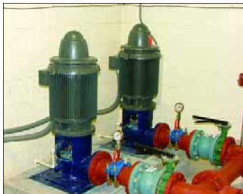
New high service pumps deliver water to the system
