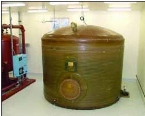
Storage tank for backwash water. After a time period to allow for settling, the cleaner water is recycled.
