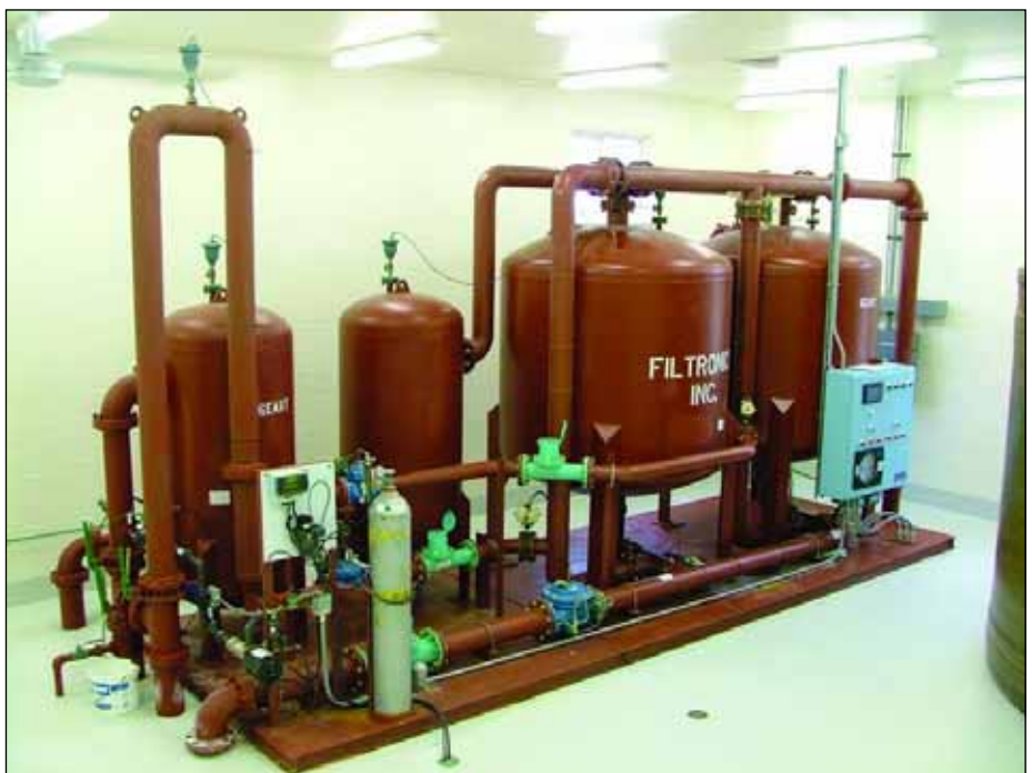
Geary RWD 4 chose the Filtronix, Inc., Dual Filter Vessel skid mounted unit. The unit seen above has two reaction tanks followed by two filter tanks.
