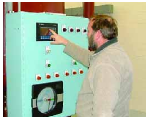
Plant operator Cliff White at the control panel is checking the display to determine the status of filter operation.
