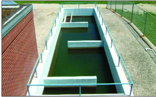
Free chlorine contact basin which provides for primary disinfection and THM/HAA control. You can also see in the upper left the metal cover to the east solids contact basin.
