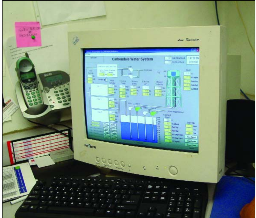
New SCADA system helps Carbondale monitor plant operations. Prior to this new system, Carbondale only had chart recorders.
