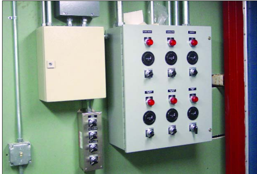
New electrical controls have been installed in Carbondale's treatment plant. The old controls were a source of many electrical problems.
