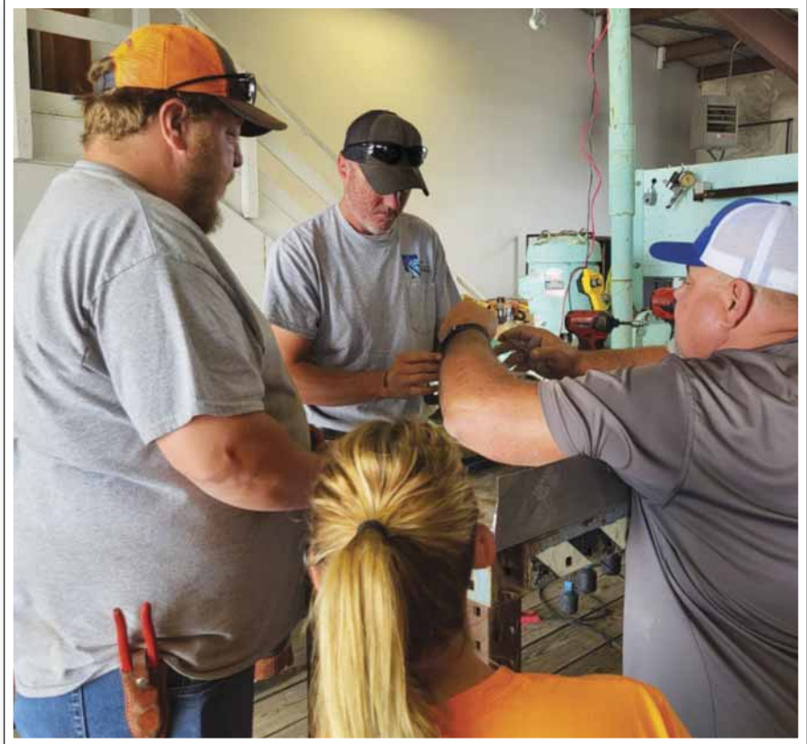
During a recent five-hour training workshop sponsored by KRWA, these operators discussed how to replace reeds in a vacuum pump. The KRWA lift station training trailer is part of the hands-on training that is being provided to wastewater operators.
