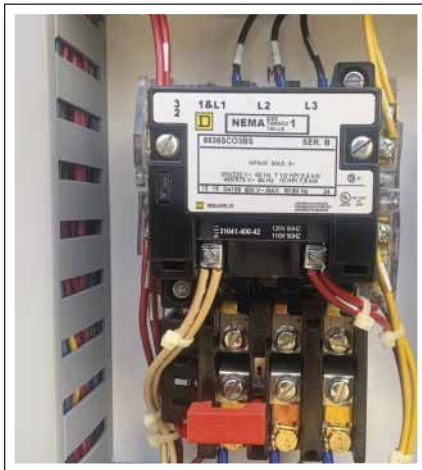
This is a typical motor starter relay commonly installed for lift stations.
