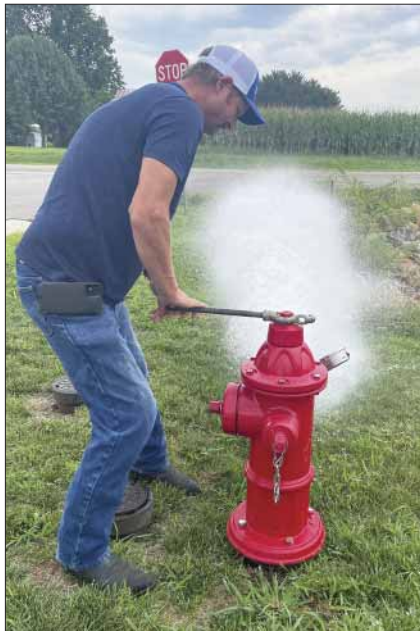
Tony Kimmi opened this fire hydrant to determine the flow rate. KRWA provides numerous hydrant tests for municipalities to help them verify information for fire insurance ratings.
