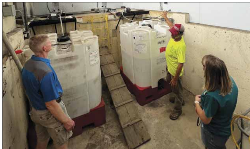
Kansas Water Office staff Kirk “TJ” Tjelmeland and Katie Goff listen to Valley Falls operator Bill McCoy as he explains chemical usage in the city’s water treatment plant. Valley Falls treats water from the Delaware River just upstream of Perry Reservoir.
