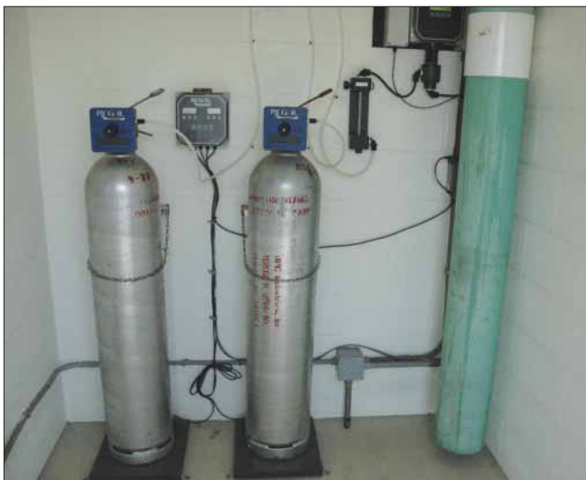
Gas chlorination is provided at the new pump station.
