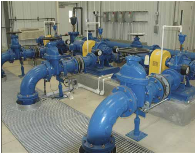
The water system improvements at Pratt included these three booster pumps at the new pump station. Each pump is provided with a 20 HP electric motor and can deliver 600 gpm to the airport 3.5 miles north of the city.
