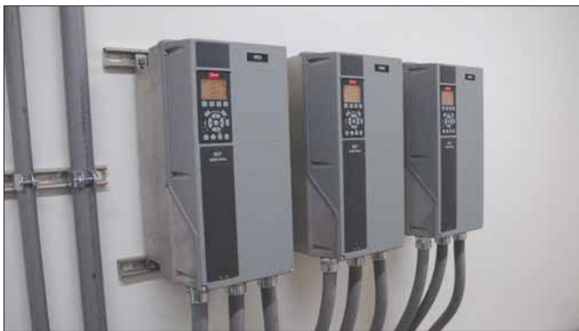
Each of the new booster pumps are controlled by a variable frequency drive (VFD). A VFD is a device that controls a motor's speed and torque by adjusting the power supply's frequency and voltage.
