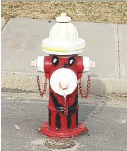
Hydrant would probably break away but it would be difficult to repair without digging it out.
