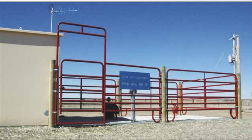
Downing Drilling of Lexington, Neb. installed this new well, No. 16. It replaces the original No. 16 well that had lost production capacity.
