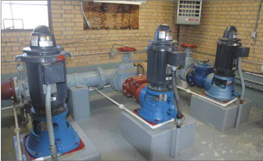
These new high-service pumps are located at the 250,000-gallon in-ground storage reservoir. All pumps on the project are equipped with VFDs.
