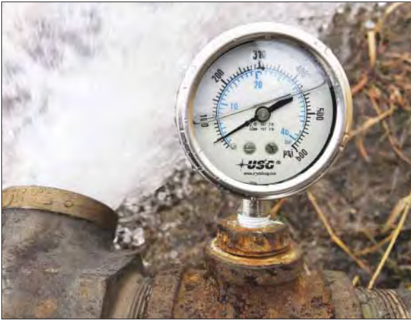
This pressure relief valve is on a fire hydrant and is set for 50 psi. KRWA has multiple relief valves for system use. Relief valves provide a safety net to help avoid pipeline breaks when a tank is out of service.
