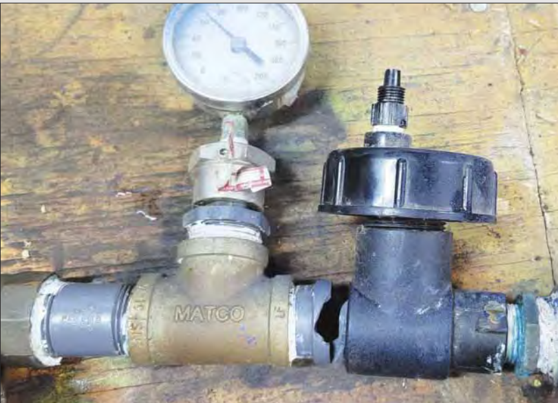
This photo shows a chlorine injector at Garden Plain that was broken due to freezing.
