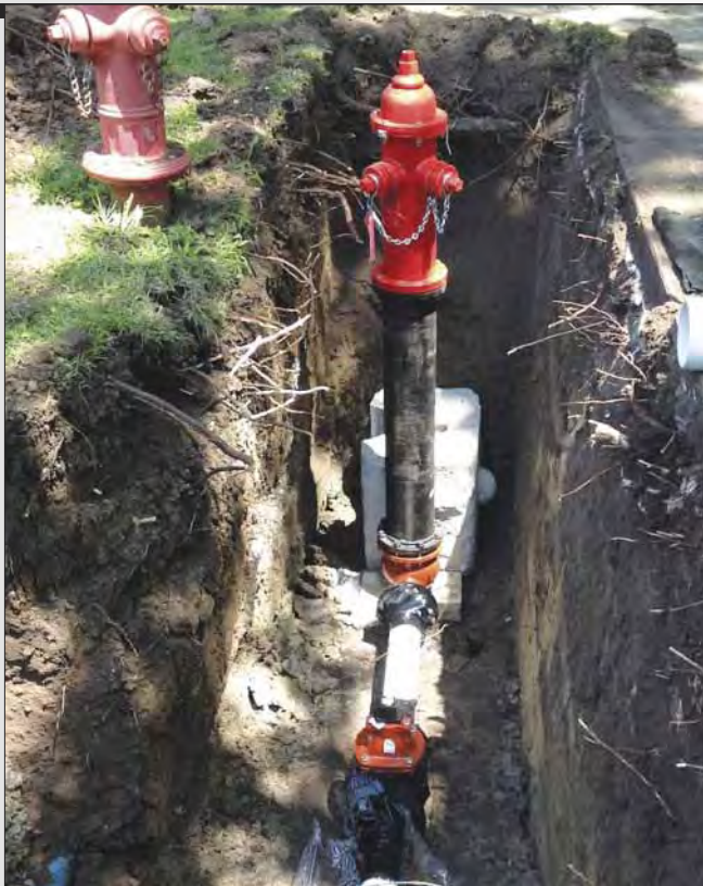
A new fire hydrant is being installed here. New fire hydrants and radio read meters were included in the project.
