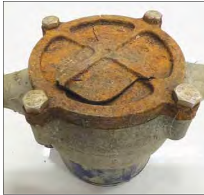
This manual-read meter froze; the meter did not register the gallons lost through the crack.
