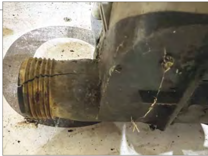
The meter had frozen; it was cracked on the inlet side.
