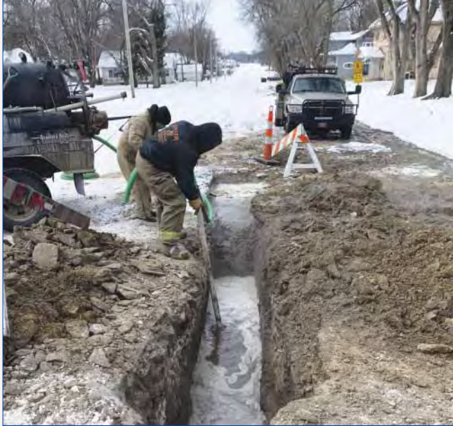
Water and wastewater system operators work in all types of conditions such as in this photo taken in a small city in north-central Kansas making a repair to a distribution system pipeline in February 2021 when the ambient temperature was -28°.
