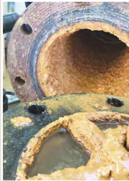
This photo shows iron deposits and bacterial growth inside the well pump discharge line.
