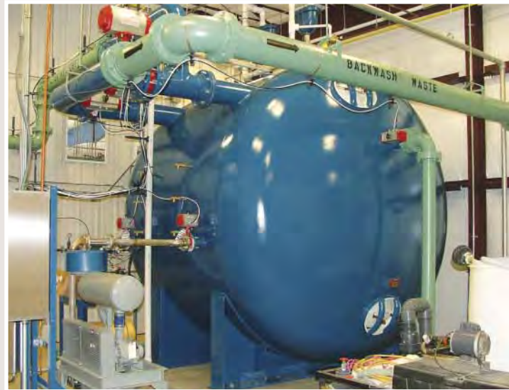
Avoid water treatment for well water if possible. First, evaluate the well for changes in water quality. This photo shows a pressure sand filter to remove iron in a rural water district plant located in northeast Kansas.
