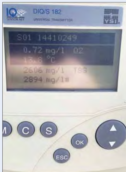
This photo show the reading from DO analyzers that control the blowers when to slow down or speed up.
