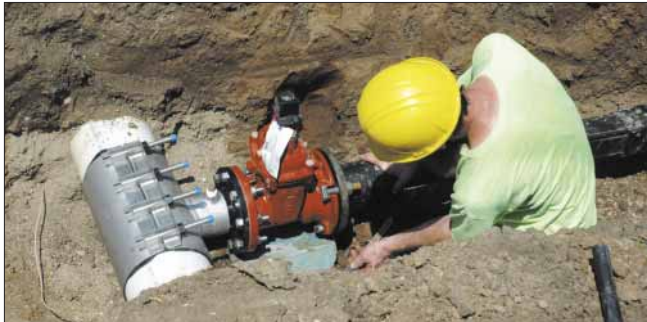
A technician with Core & Main, Wichita, demonstrates making a live tap. A 4-inch line is being tapped into an 8-inch water main serving the industrial section of town.
