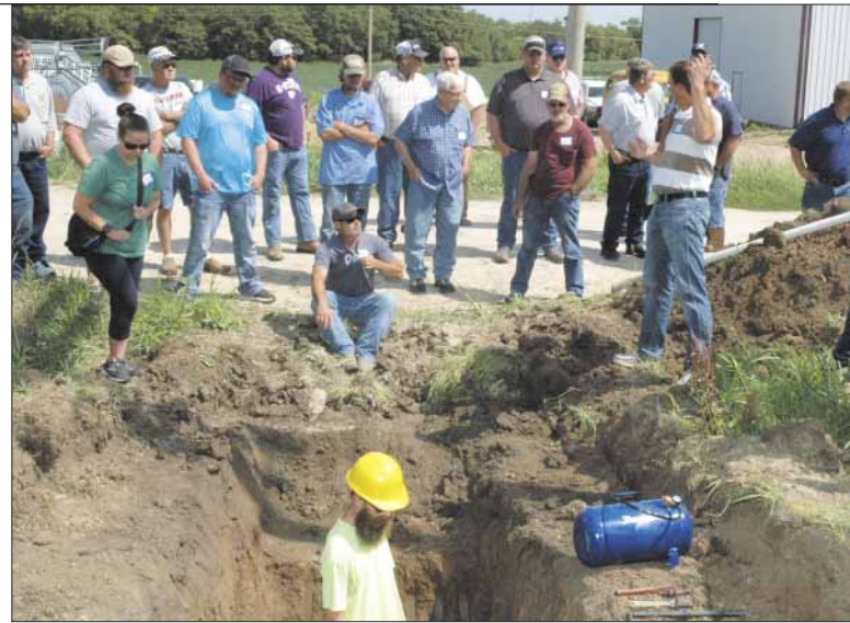
Attendees moved to the field to observe a live water line tap.
