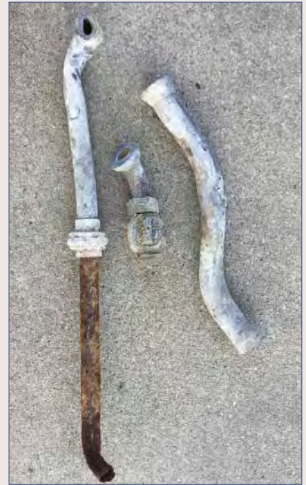
This photo shows lead piping from a service connection line gooseneck that connects the water main to a residential water meter. This particular piping came from a small city in central Kansas that replaced all city water lines, all city service connection lines, and water meters.
