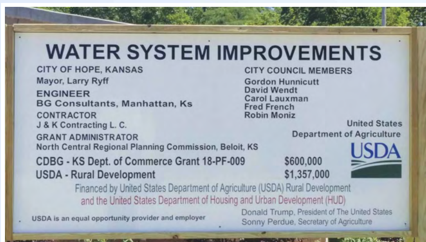
A "project sign" is required when Kansas Dept. of Commerce funding is involved.
