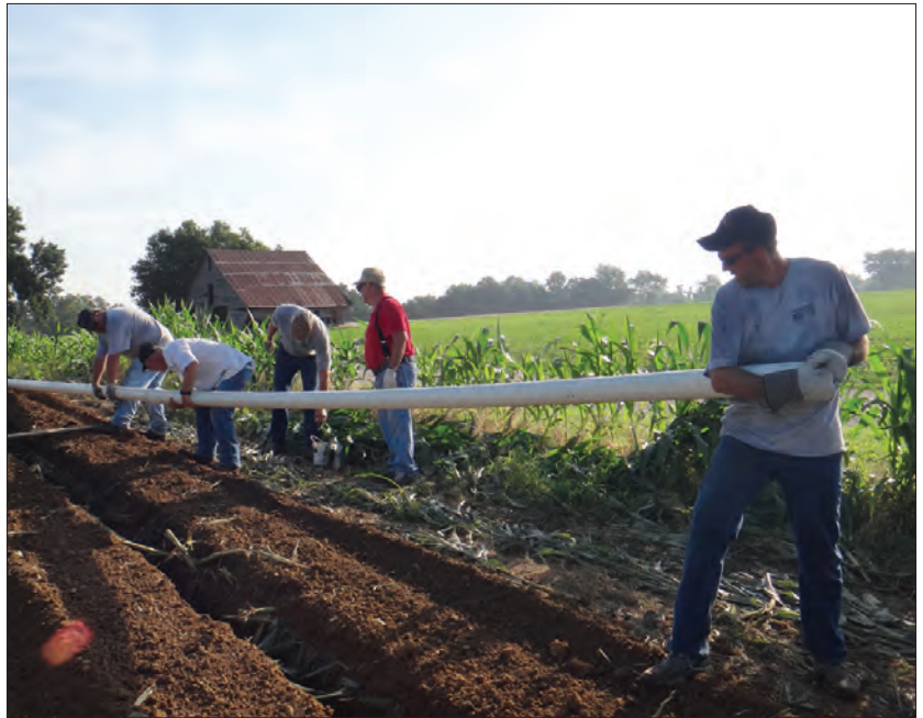
Volunteer Ken McNickle says, "Hold it steady, I'm trying to push." Ken is pushing one pipe to connect it to the others that have already been assembled. Those holding at the assembled end are George Katzer and Clayton Merrick. Rod Brimm is getting more lube for the next joint while Sam Atherton is looking on. This is at the north end of the 700 feet of trench in the cornfield rounding the bend. This is the second of three projects started June 26, 2013 and June 27, 2013.
