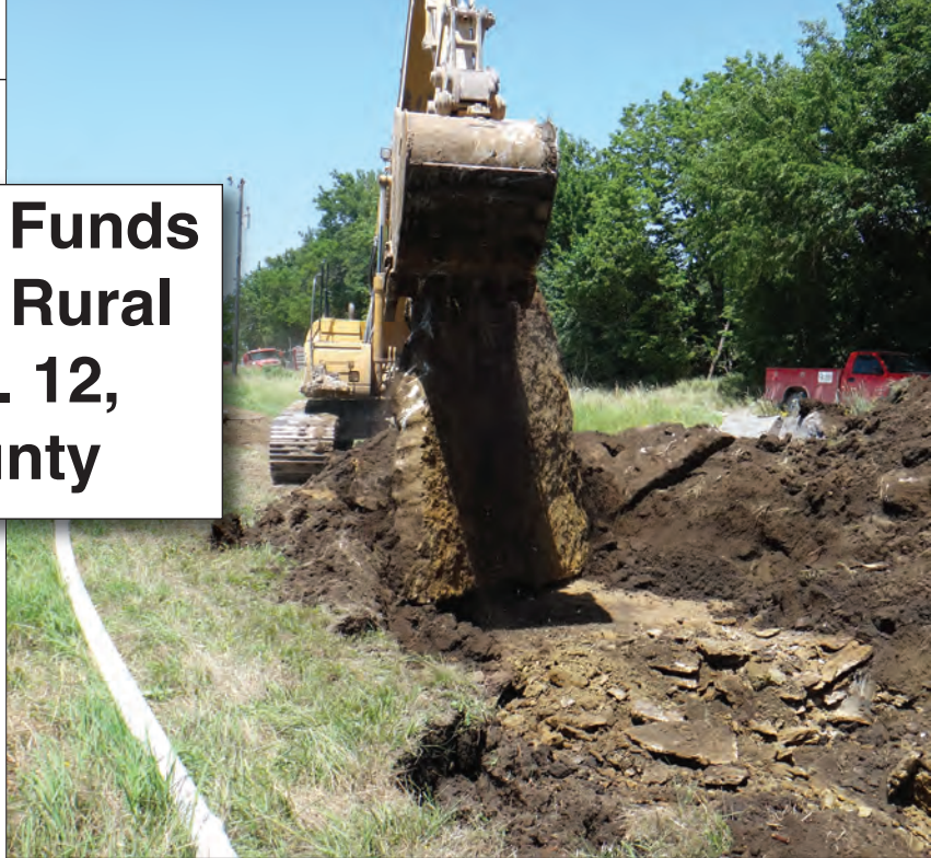
Big Rocks! Volunteers had to remove very large rocks found in their path on the second project on Reno Road. They had to stop and spend several days working on the rock before they could finish trenching and laying the new 4-inch line. Jackhammering was done July 3, 2013 and July 10, 2013.
