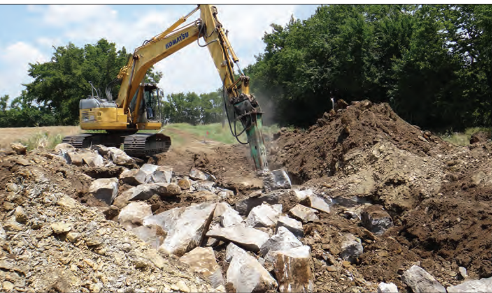
A jackhammer will help! The operator on this backhoe prepares to break up some rock. This had to be done to be able to remove the rock and open the area up to lay the pipe. This was the second of three projects started July 3, 2013 and July 10, 2013.
