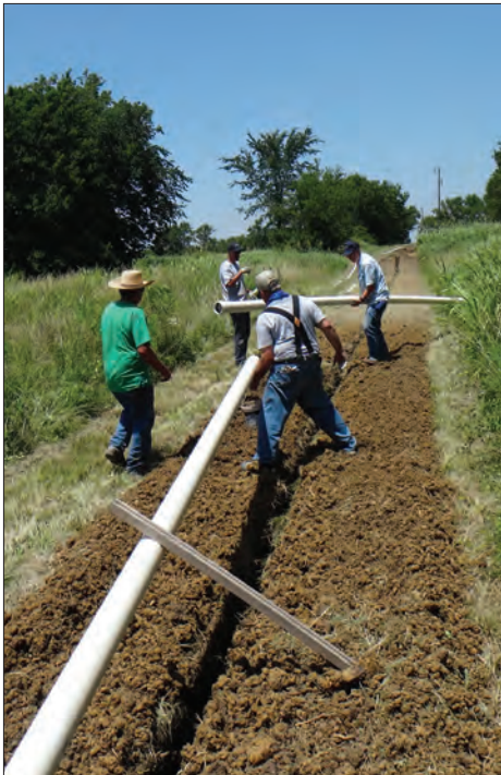
More 4-inch is installed. Sam Atherton, Kerry Bright, George Katzer and Rod Brimm connect the new 4-inch line and place it in the trench. This is the second project started June 26 and June 27, 2013.
