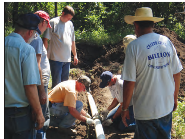
Four hands are better than two. Steve Lumbley, on left, and Ken McNickle, right, assemble a bell restraint on the new 4-inch main. Watching to learn how this is done are: (left) George Katzer, Don Brothers, Bill Foster. Kerry Bright is to the right. This work was on CR 5800 on June 12 and 13, 2013.
