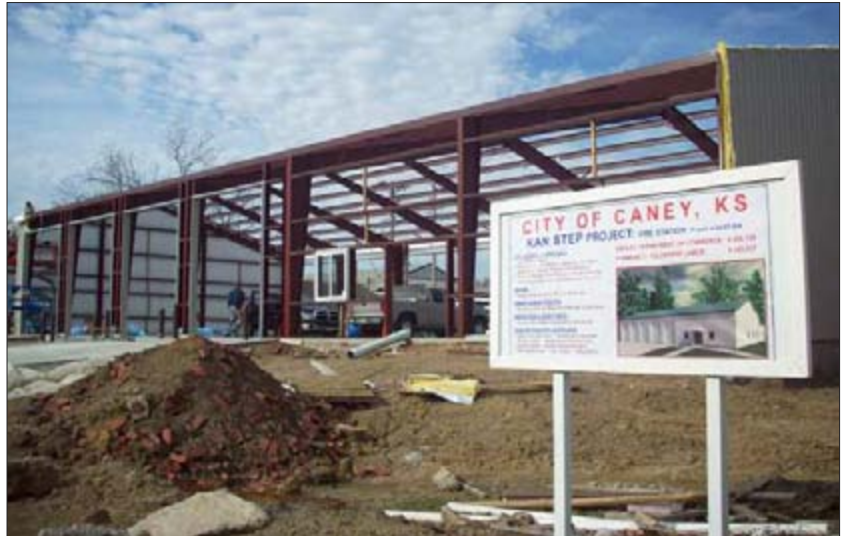
This photo, taken in April 2011, shows the framework of the new KAN STEP fire station in Caney, KS.
