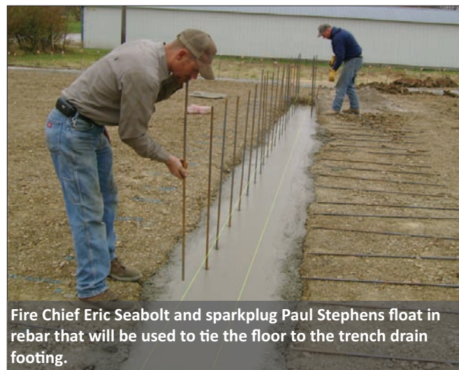
Volunteers Steve Flora and Bob Hearn bend 3/8-inch rebar which will become column stirrups that will encompass the main column anchor bolts on the fire station in Sawyer.
