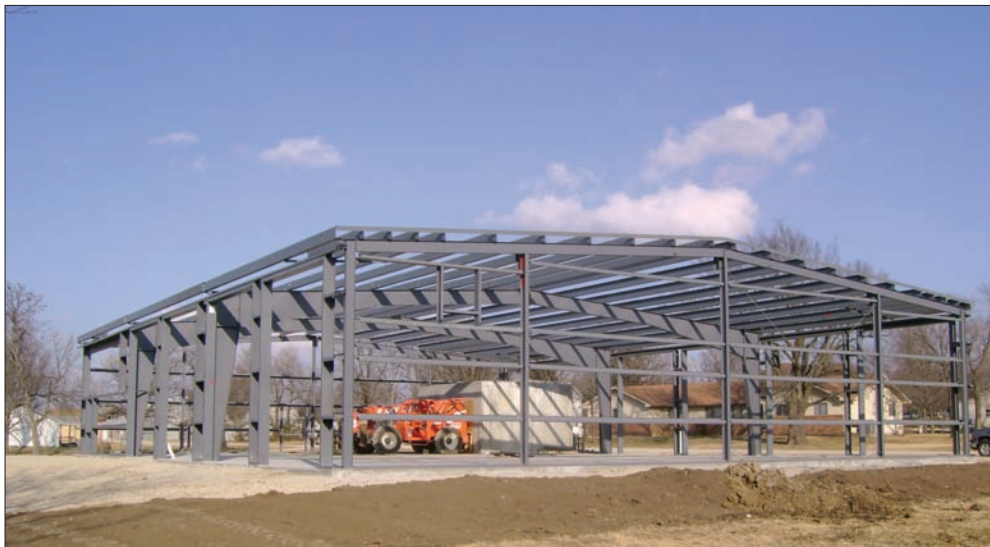
This photo shows the Anderson County Fire Station as it appeared on Dec. 30, 2010. D & B Collaborative, Lawrence, KS, is overseeing the erection of the building by Heinen Custom Operations, Valley Falls, KS. Anderson County is paying for the erection of the building.
