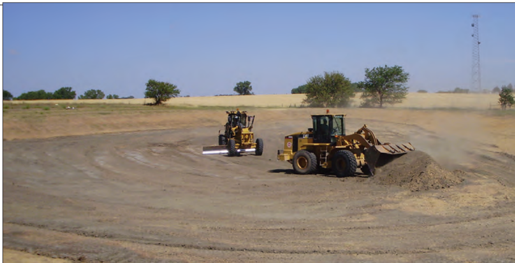
A grader is used to gather debris off the bottom of the lagoon cell. The debris can include wind-blown dirt and minor amounts of sludge and dead vegetation. Such material will prevent good compaction. In addition to the grader, a front-end loader and dump truck are used to remove the debris.
