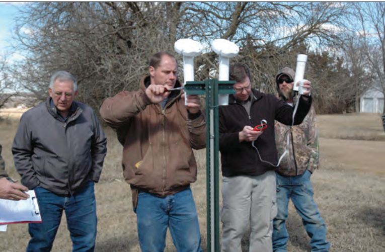
District Operator Jeff Schlabach works at installing a satellite meter reading unit during a demonstration sponsored by IDT and the RWD.
